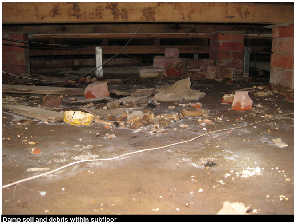
Damp soil and debris within subfloor
