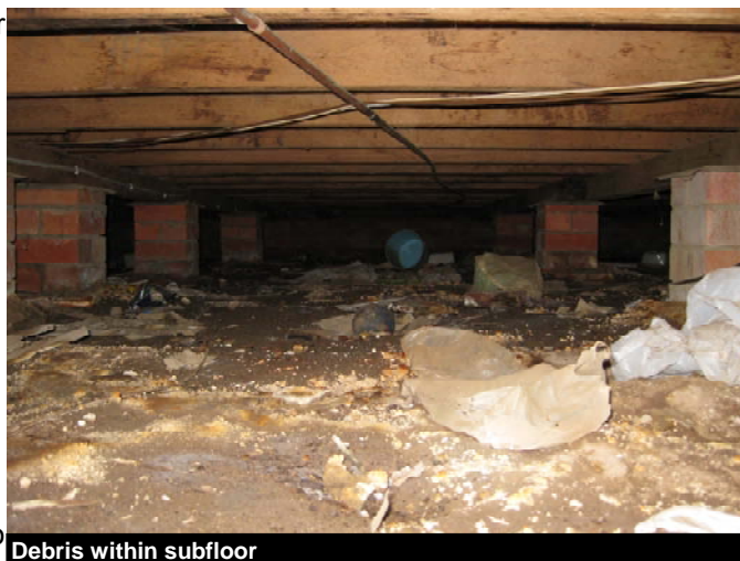
Debris within subfloor
