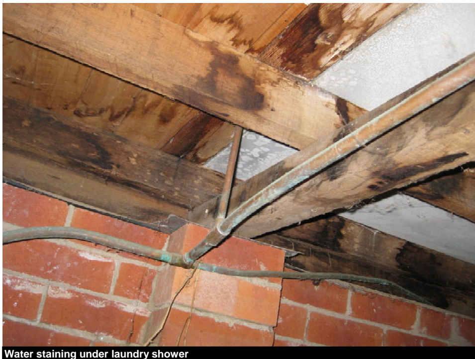
Water staining under laundry shower
