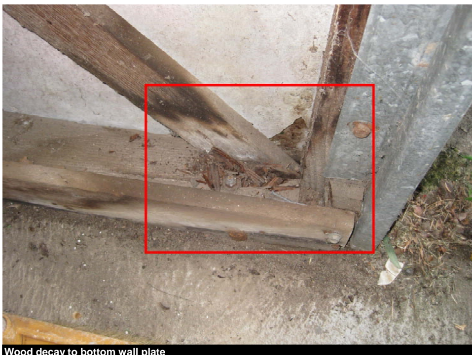
Wood decay to bottom wall plate
