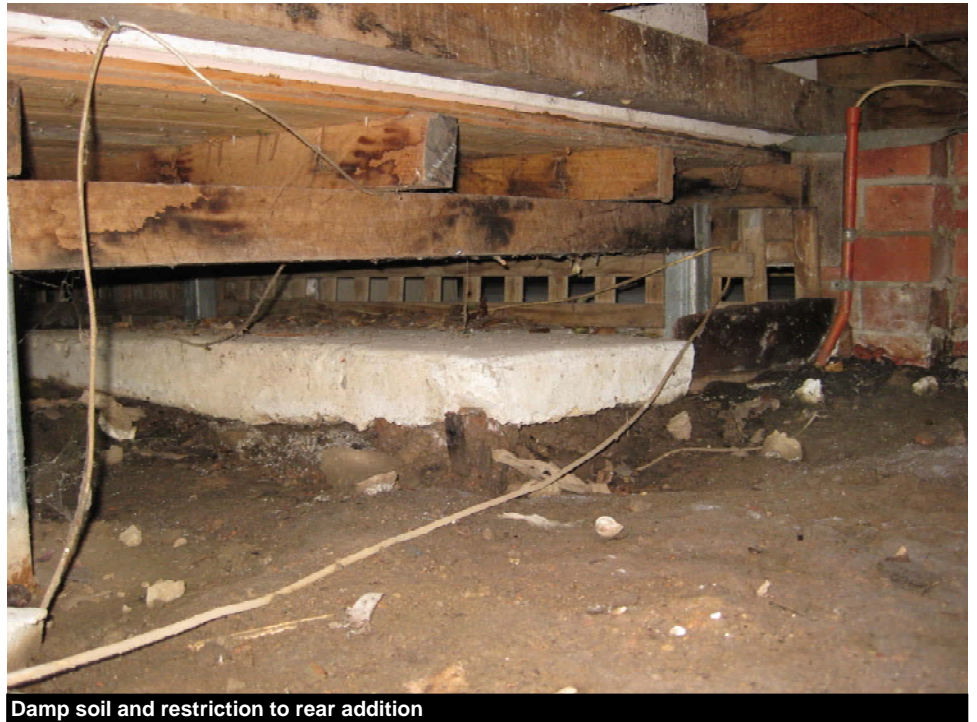
Damp soil and restriction to rear addition
