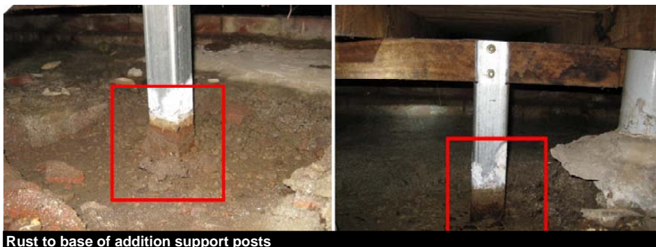
Rust to base of addition support posts
