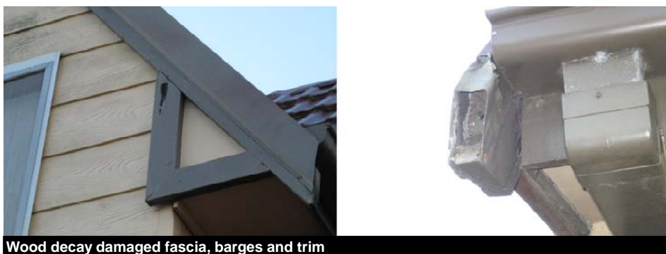
Wood decay damaged fascia, barges and trim
