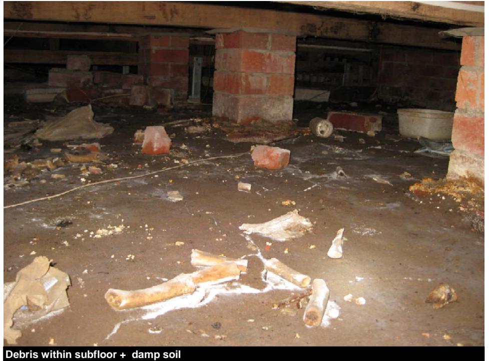
Debris within subfloor + damp soil
